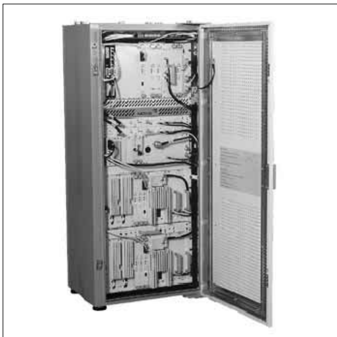
Base station of cellular network
